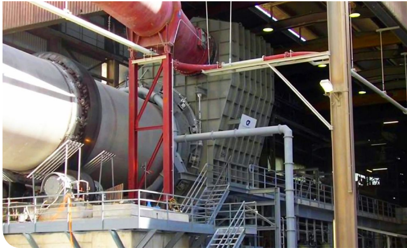
The ETA Cooler at the Holcim Untervaz Cement Plant in Switzerland is a huge machine that’s almost half a football field in size. Courtesy of Claudius Peters.
